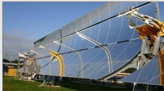
Test facility PCS
